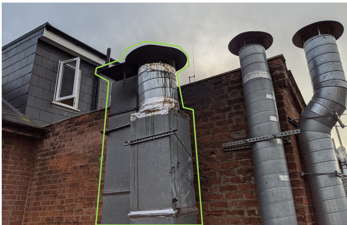
Figure 5.1 – Premises fan ducts
