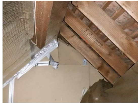
20. Gap over boarding at apex of front gable end.
