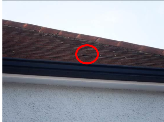
4. Slightly lifted roof tile (southeast elevation).
