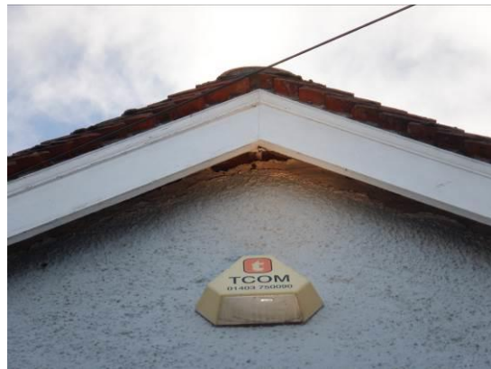
6. Gap at apex of front gable end (front elevation).
