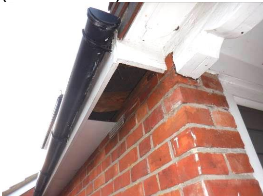
11. Large hole in soffit leading into garage (southeast elevation).
