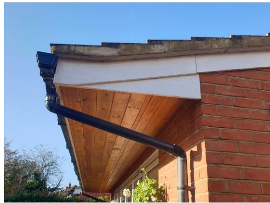
14. Tight timber barge boards and rear overhang.
