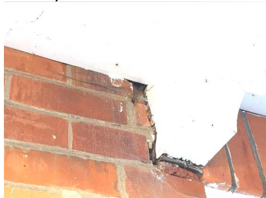
10. Cobwebbed gap into brickwork around porch roof timber (front elevation).
