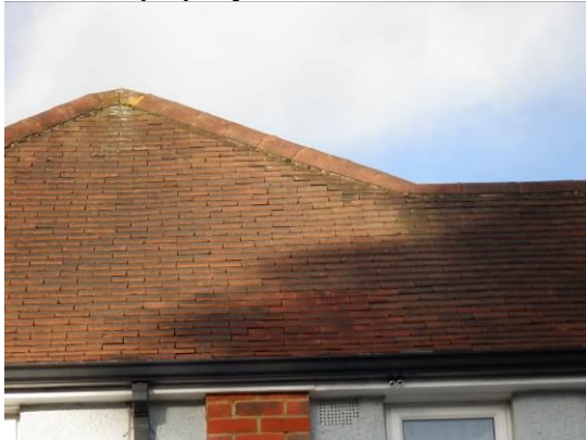
3. Raised roof tiles adjacent to roof hip (rear elevation).
