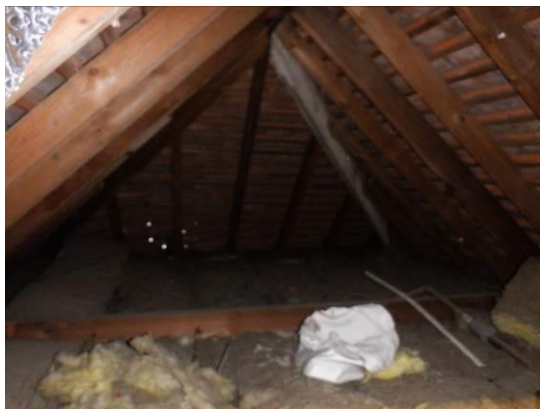
17. Unlined roof in southeast-facing hipped end.
