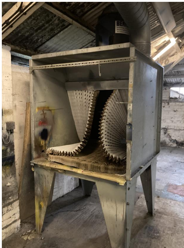
Plate 11: View of extractor unit within industrial (rear) building.
