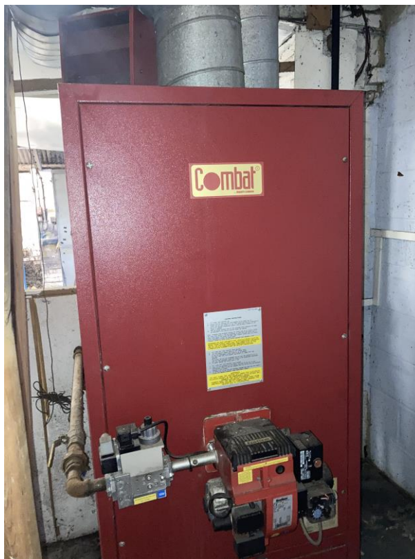
Plate 9: View of industrial heater within industrial (rear) building.
