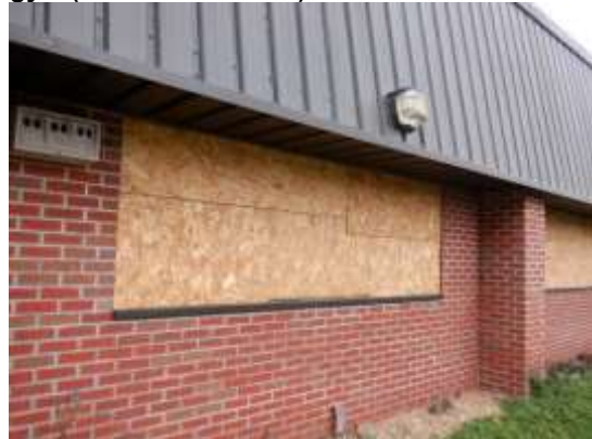
4. Gym windows sealed with OSB (northern elevation).
