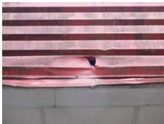
8. Puncture in metal cladding (northern elevation).
