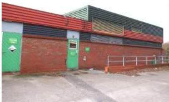
11. Broken vent on door to electrical store (eastern elevation).
