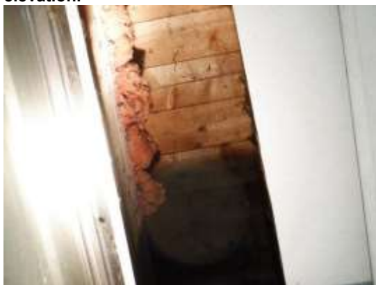
9. Missing ceiling panels above rear entrance to sports hall (northern elevation).
