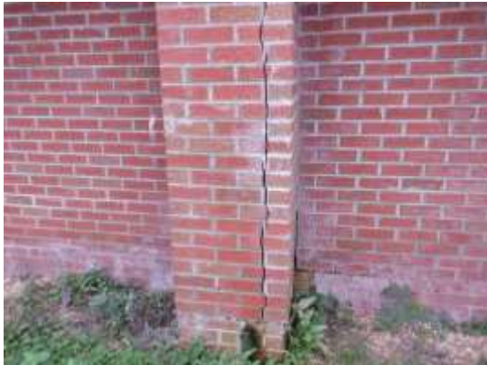
3. Crack in gym brickwork (northern elevation).
