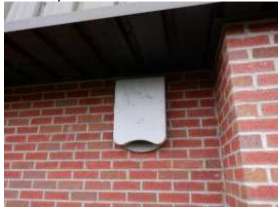
6. Bat box with bird droppings (northern elevation).
