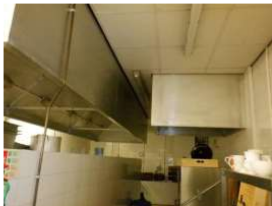
20. False ceiling tiles in kitchen.
