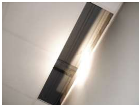
18. Missing ceiling tile in gym.
