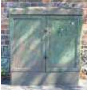
Cast iron cabinet
