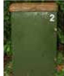
Single door cabinet (with replacement steel door)
