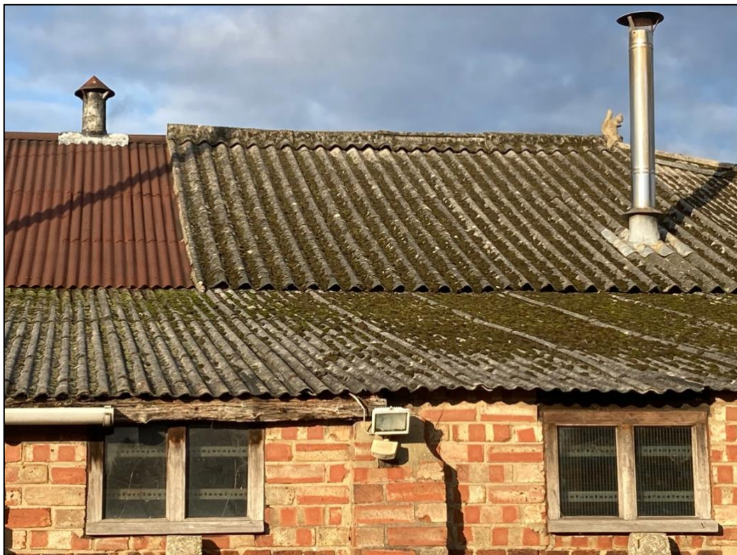
Photograph 10. The southern aspect of the workshop roof with a gap created where the chrysotile roofing sheets meet the ridge.
