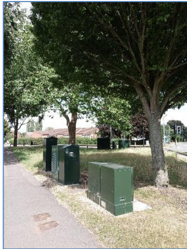
Fig 7. Existing cabinets next to proposed equipment location.
