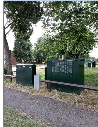
Fig 9. Existing cabinets to the south east corner of the grass verge.
