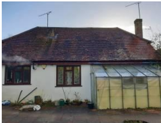
2. The rear elevation of the bungalow (B1), featuring a hipped roof with broken and lifted roof tiles.
