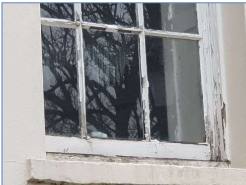
Fig 3. Rear window, deteriorated condition.
