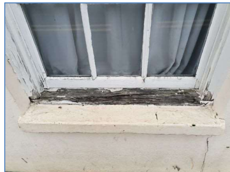
Fig 4. Street window, deteriorated cill detail.
