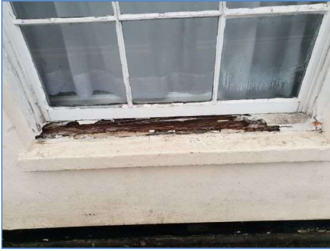
Fig 5. Street window deteriorated cill detail.
