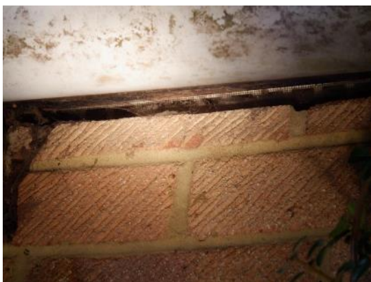
7. Tight vented soffit along eaves of the house, flush to the brickwork.
