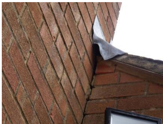
12. Lifted lead flashing on rear elevation where the garage joins the house.
