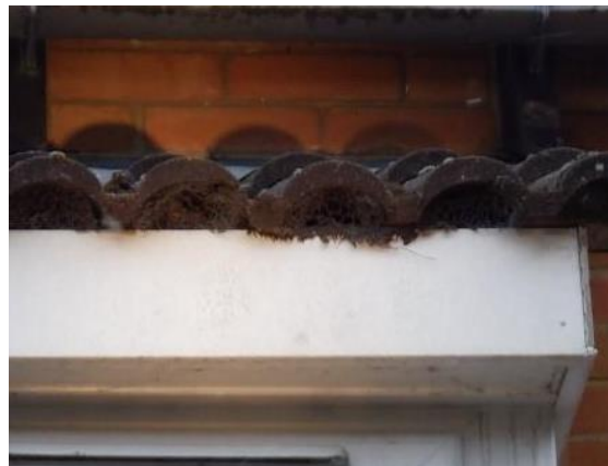
6. End of roof tiles above bay window covered in chicken wire.
