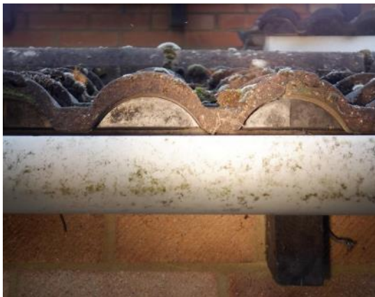
5. End of roof tiles blocked on side extension.
