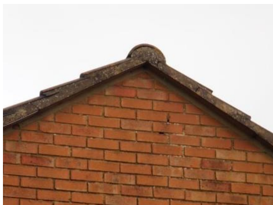
8. Intact mortar and under cloaking tiles on verge of the main roof.
