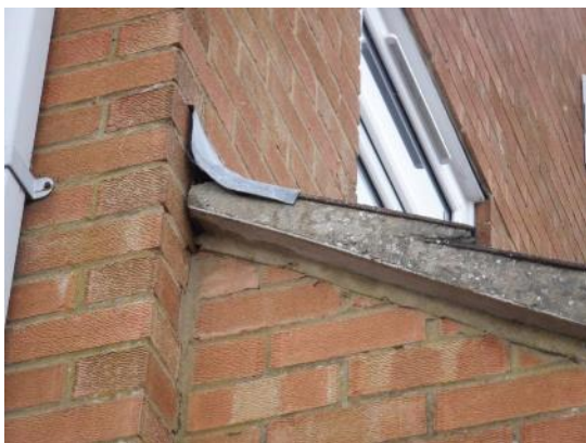
11. Lifted lead flashing on the eastern elevation of the porch roof.
