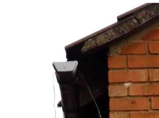
9. Broken mortar under verge tile on the south-eastern corner.
