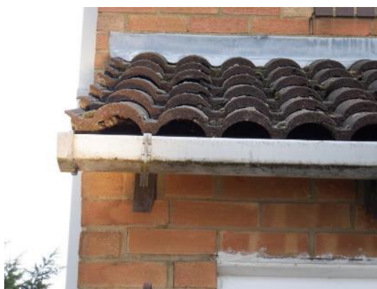
10. Unblocked verge tiles on porch roof on the front elevation.
