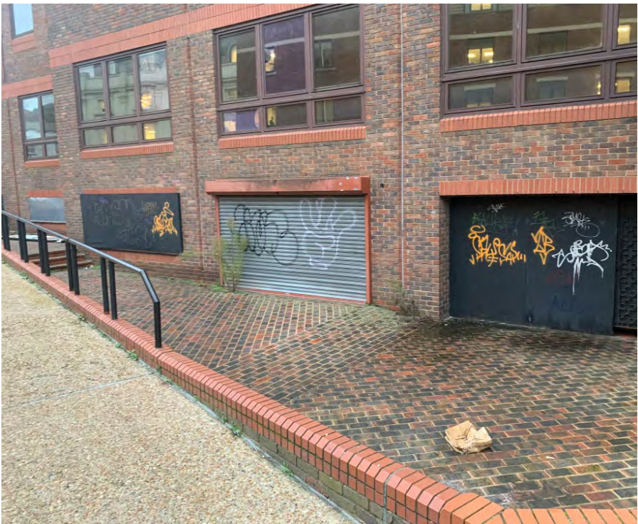
5. View from the ramp showing the poor conditions surrounding it
