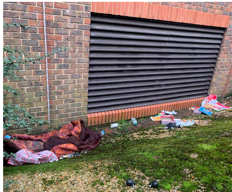
2. Sleeping beds and dumping zone behind substation high walls
