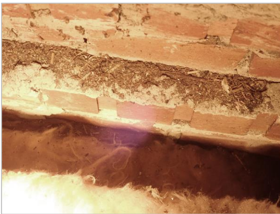
Photo 9 Brickwork at base of partition wall (debris but no bat droppings)
