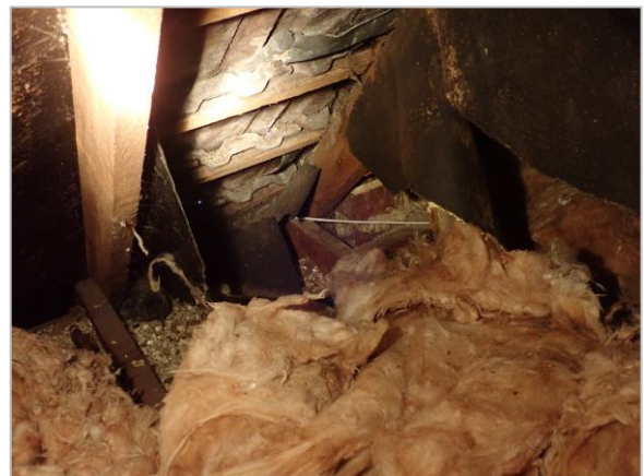
Photo 12 Section of damaged felt
