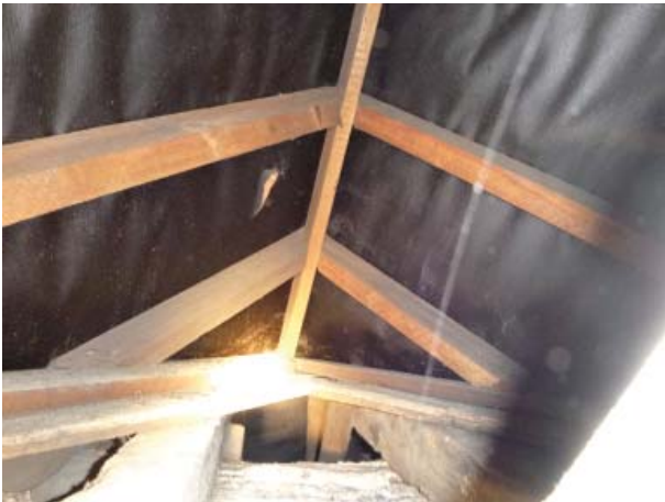
Plate 9. Roof void above dormer window on third floor of of 27-28 Market Place - 'Kik Sports'. Small tear in bitument felt lining. Visible via hole in ceiling.
