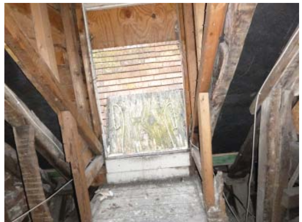
Plate 18. Chicken wire over window in roof void of 29-31 Market Place 'Coopers Arms'
