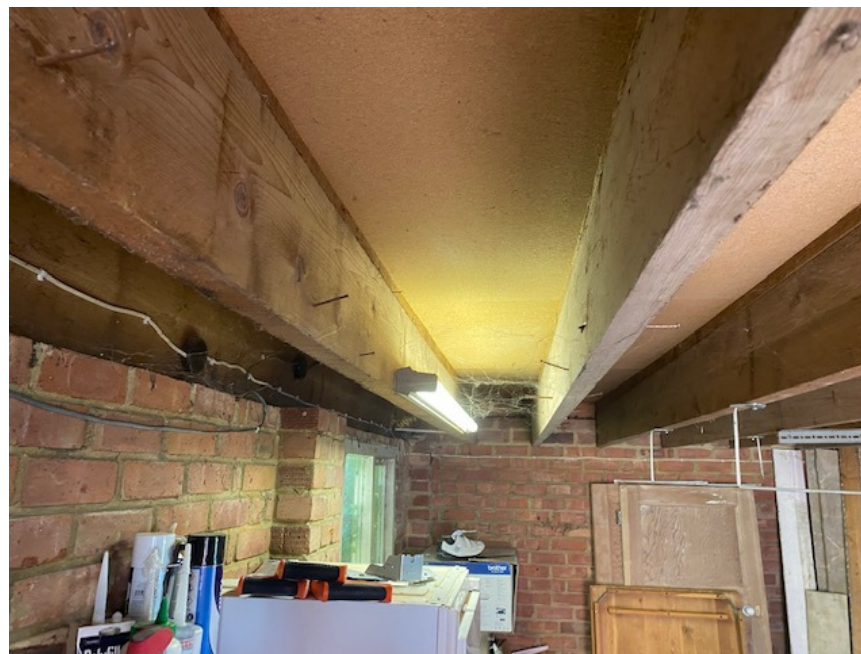
Photo. 4 Cobwebs between every joist and open joists reducing tighter gaps favoured by local bat species
