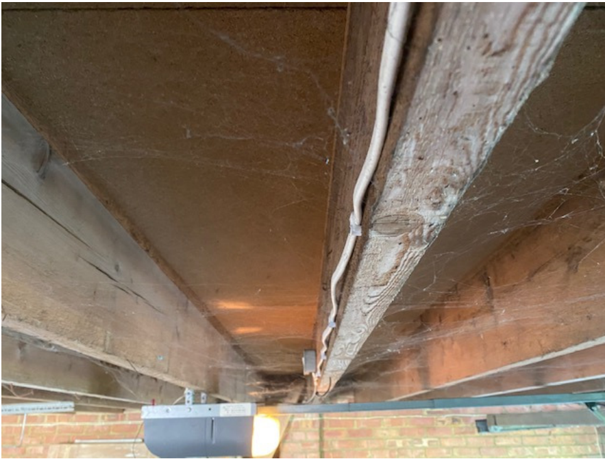
Photo. 1 Extensive cobwebs between every roof joist
