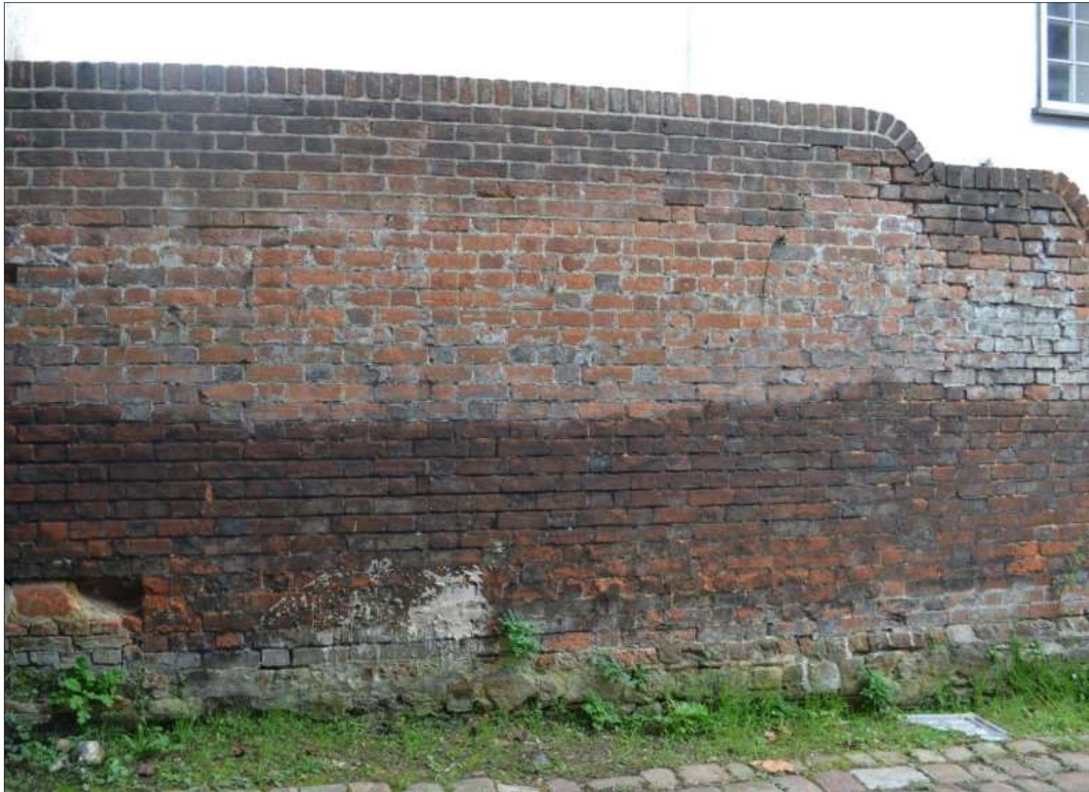
Figure 19: Northern section of the wall - note the missing bricks along the lower courses, evidence of efflorescence & open mortar joints where inappropriate cementitious mortar has fallen away.
