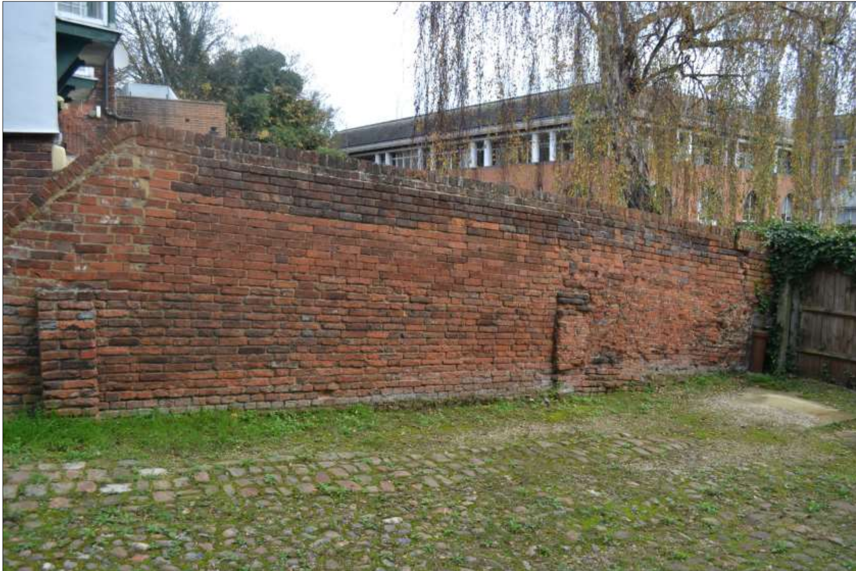
Figure 14: Southern section of the boundary wall - note the various phases of repair and low-level buttresses
