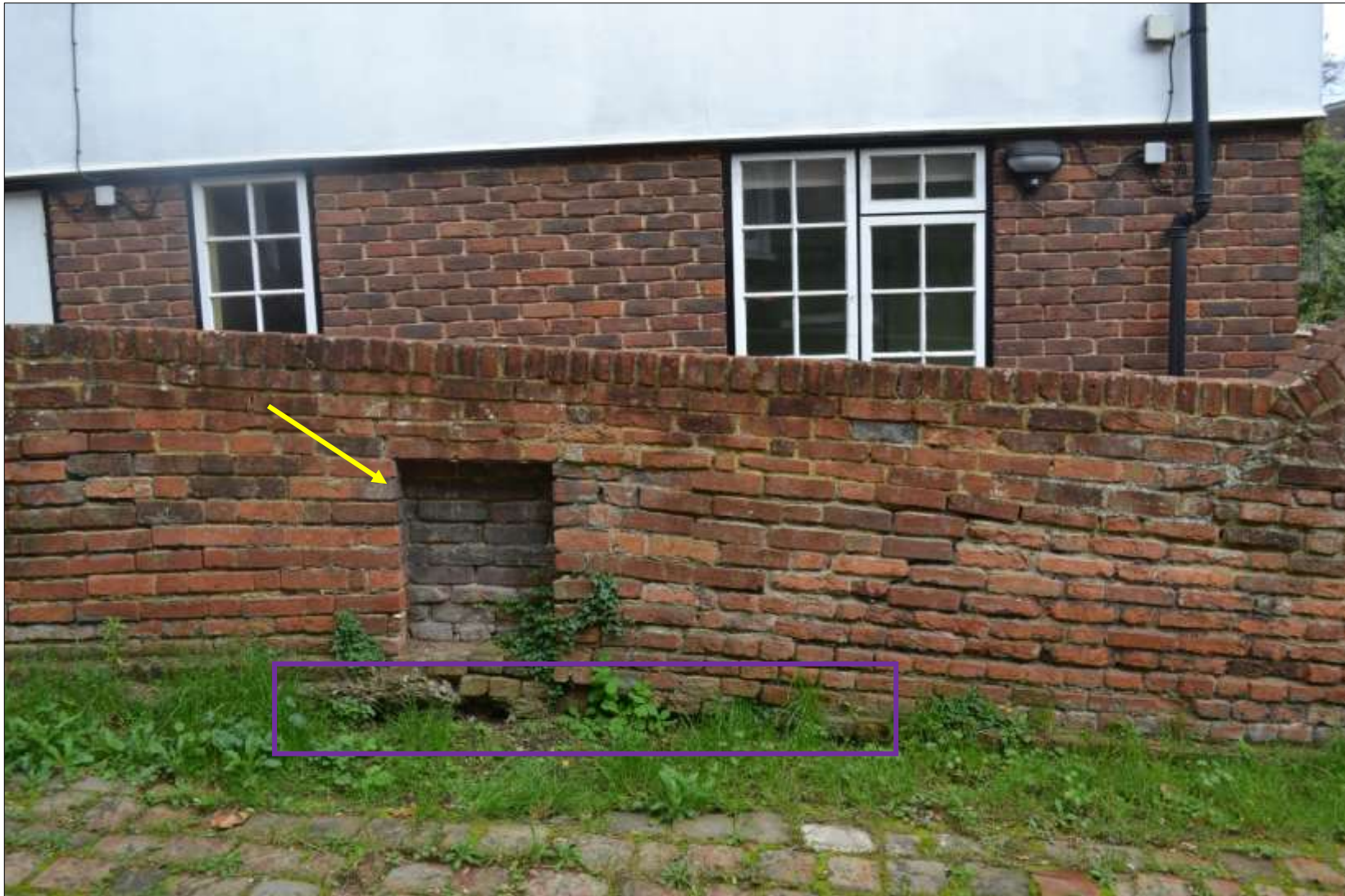
Figure 18: Middle section of the wall - note the missing buttress, highlighted in yellow, and missing bricks along the lower courses highlighted in purple
