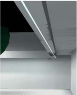
Continuous LED strip lighting inside canopy
