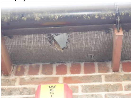
21. Tear in roofing felt at the eaves on the northern side of the pavilion (B1)
