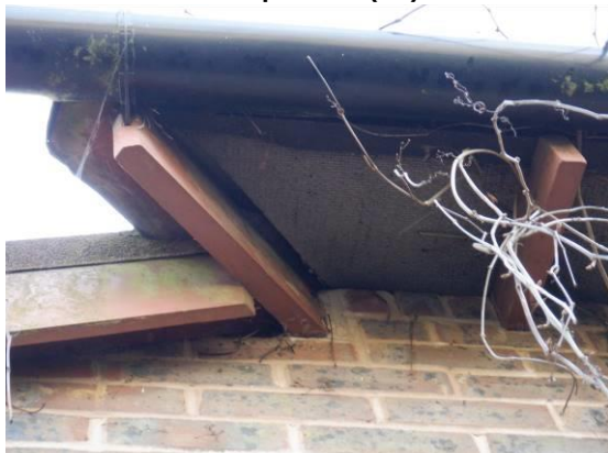
23. Gap on the central hipped roof at the northern side of the building where the hipped roof and eaves joined the brickwork
