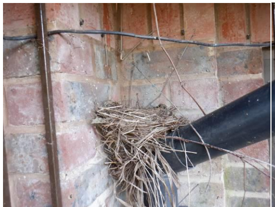
22. Bird nest on some guttering towards the northern side of the pavilion (B1)
