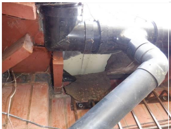
20. Tear in roofing felt at the eaves on the northern side of the pavilion (B1)
