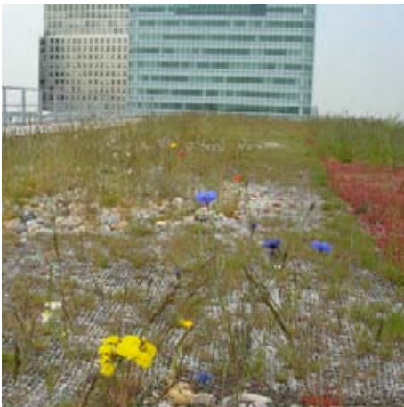
Figure L45: Biodiverse green roof
