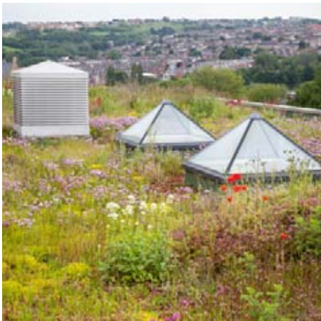
Figure L46: Biodiverse green roof
