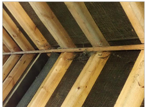
Photo 12 Ridge and roofing felt
