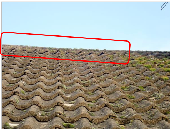
Photo 15 Slight gaps to tiles to left hand side of front elevation
