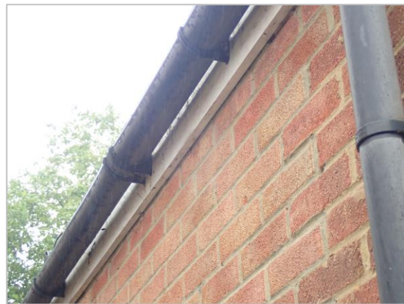
Photo 16 Fascia around flat roofed extension
