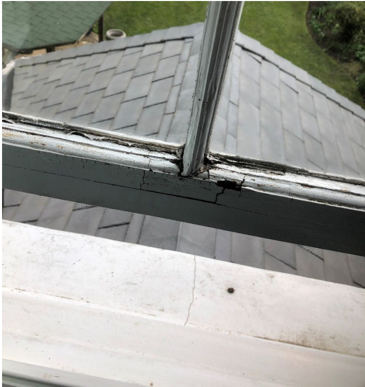
Bathroom sash bar
