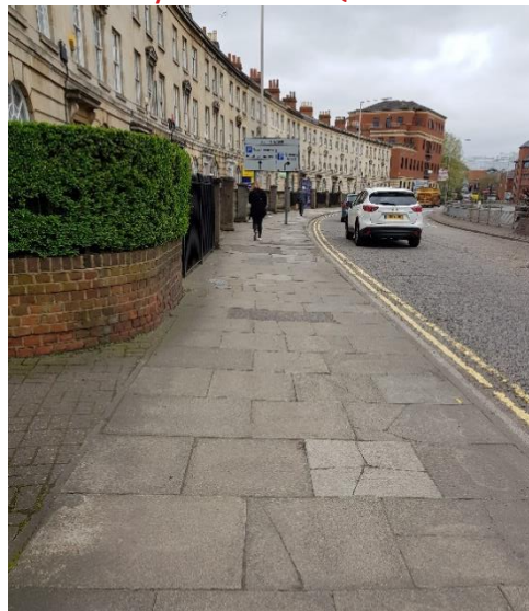
Figure 2.3. Footway Conditions on Queen's Road
