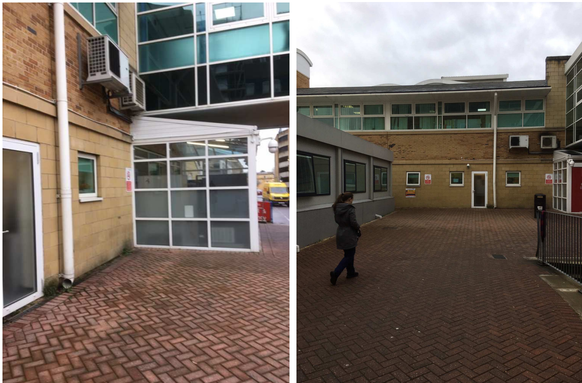
Figure 5: Photos demonstrate locations of existing external condensers.
