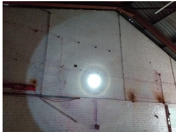
13 - PRF 2 gaps in the brickwork leading to cavity space.
