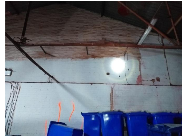
11 - PRF 1- gaps in the brickwork leading to cavity space.
