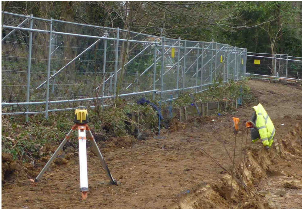
Figure 6. Photograph extract from FLAC site visit 01.03.17 to show position of former shallow retaining structure opposite 3030 to 3031, diminishing opposite 3029
