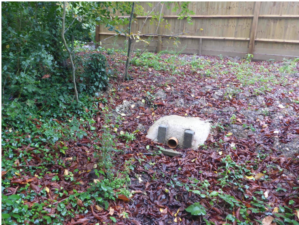
Figure 8. Land drain discharge located within RPAs of 3047 and 3048
