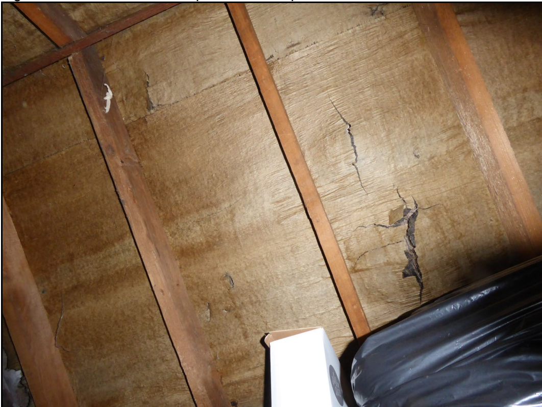
Figure 11. Membrane in loft space. 33 Hilltop Road, Caversham. 28.06.21
