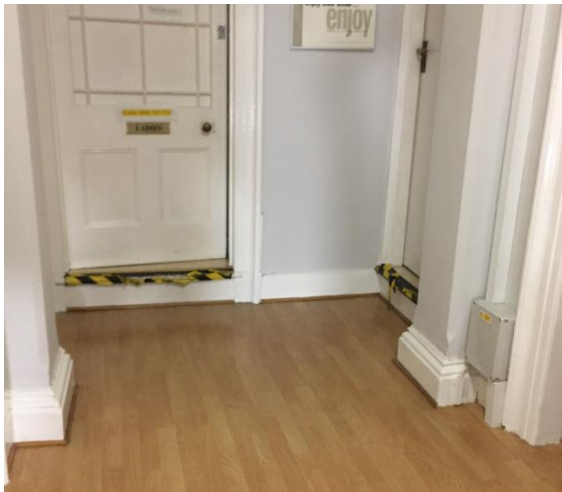
26. Inconsistent skirting by WC
