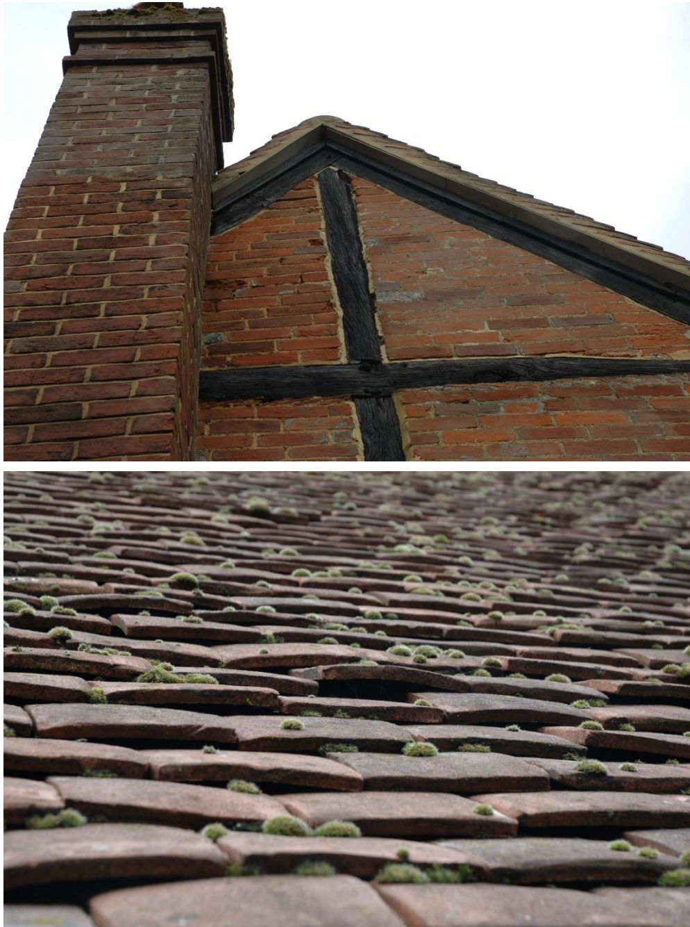
Figure 4.9 Example of potential bat roosting features on building 3 – gap between brickwork and wooden beam (above) and gap beneath roof tile (below)
