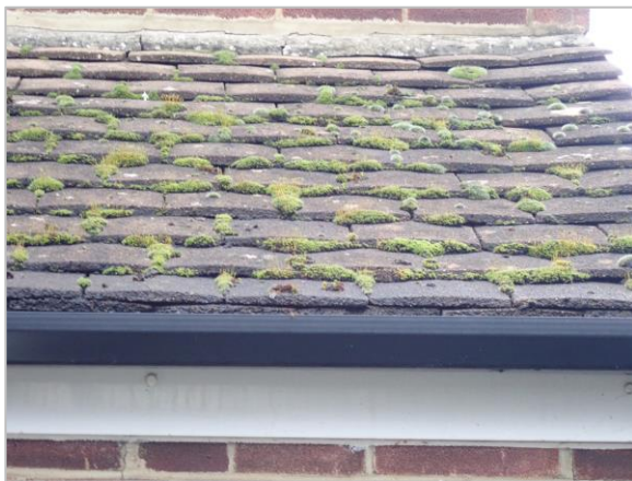
Photo 15 Roof tiles to small rear single storey extension
