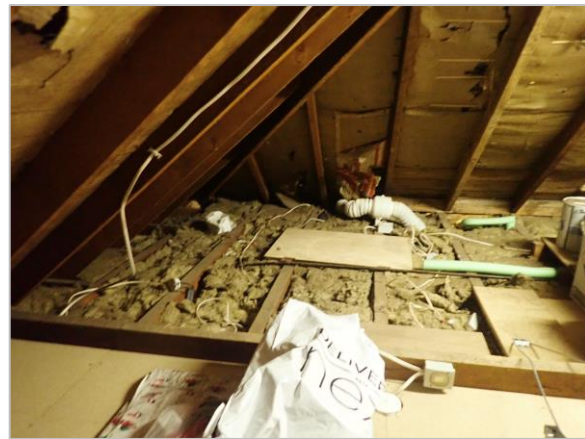
Photo 4 General conditions in main loft southern hip gable end)
