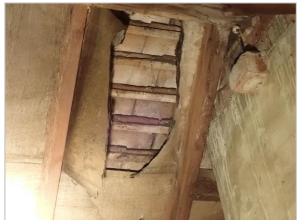
Photo 12 Damage to felt showing underside of tiles
