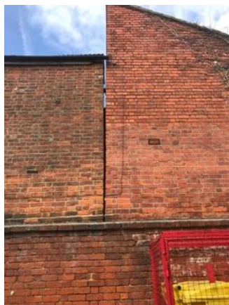
Photograph 5: Gaps between the walls of the two sections of the building
