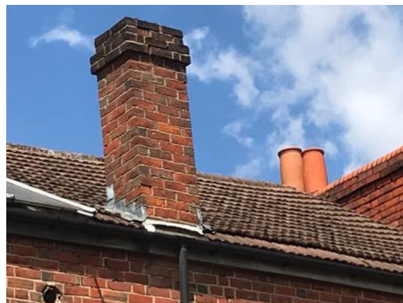
Photograph 6: Raised tiles on the southern elevation
