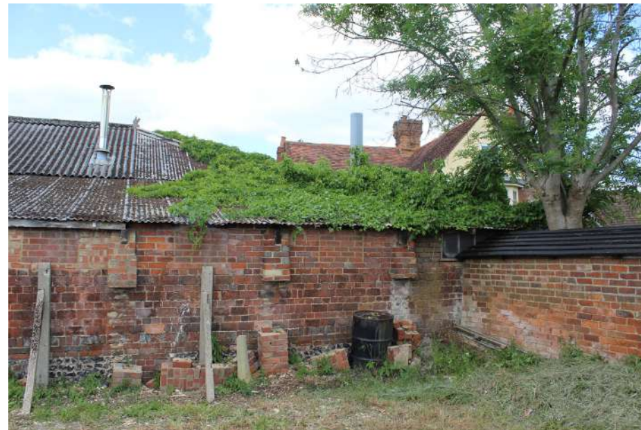
South elevation of 389 Gosbrook Road workshop, with rear wall in a poor state of repair. Ivy Farmhouse rear elevation beyond
