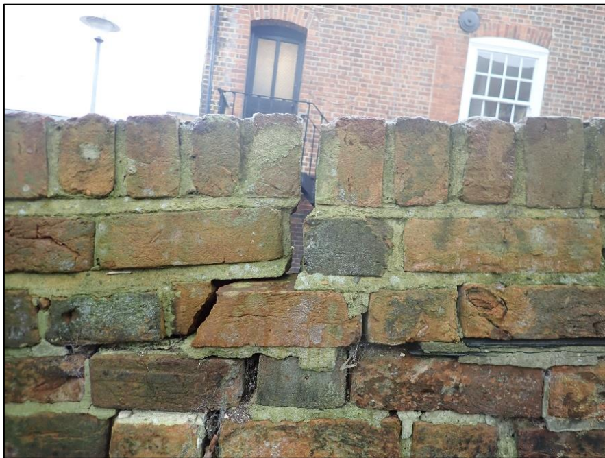
Figure 21. View of the crack at the top of the wall from No. 15.
