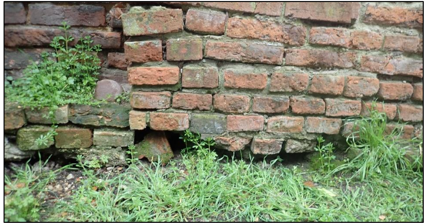
Figure 14. Undermining of wall.
