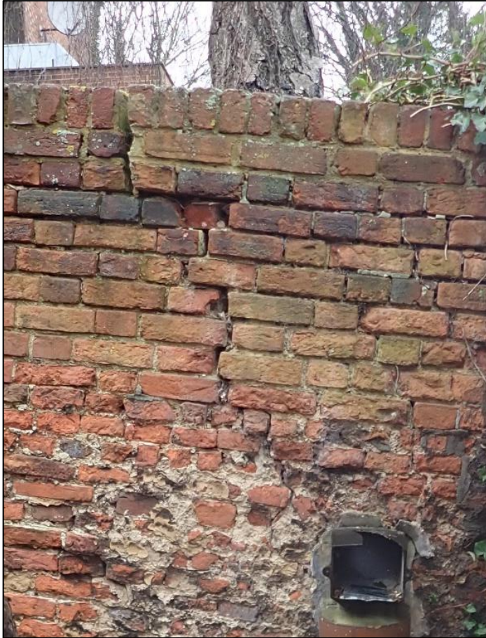
Figure 17. Tapered, vertical crack at the south end of the wall.
