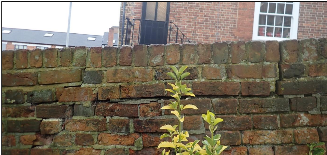
Figure 23. Loose brickwork to the north of the crack.
