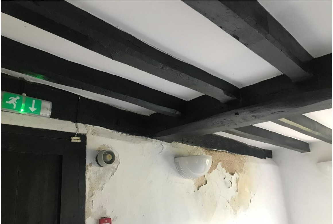
Figure 35 Exposed timber framing to ceiling in north ground floor room. Note damp at head of wall.
