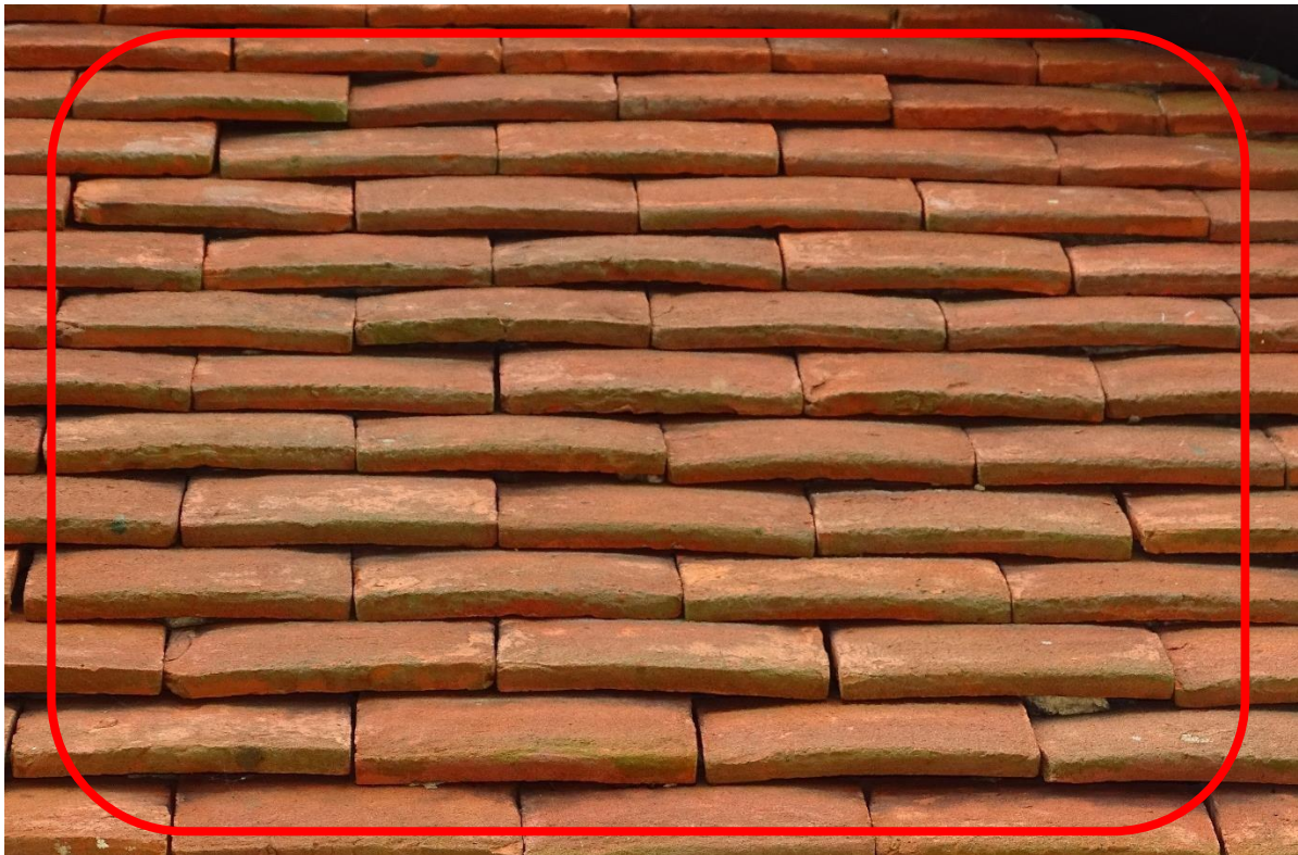
Image 2 – Gaps within the vertical tiles to the East facing elevation which offer access value to bats within
