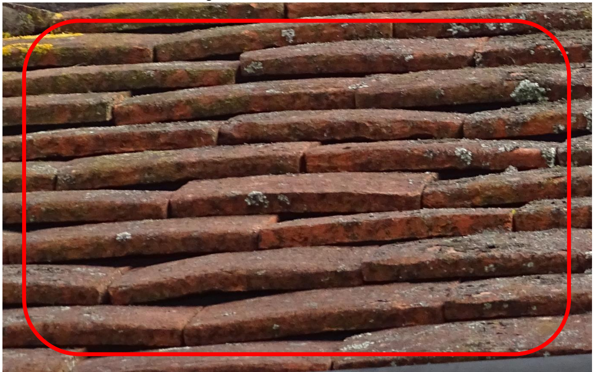
Image 7 Gaps within the West facing roof coverings which offer access values to both crevice & void dwelling bats
