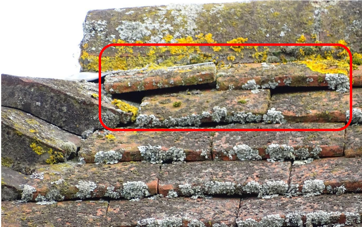
— Image 6 – Gaps below the ridge tiles which offer roosting value to bats within
