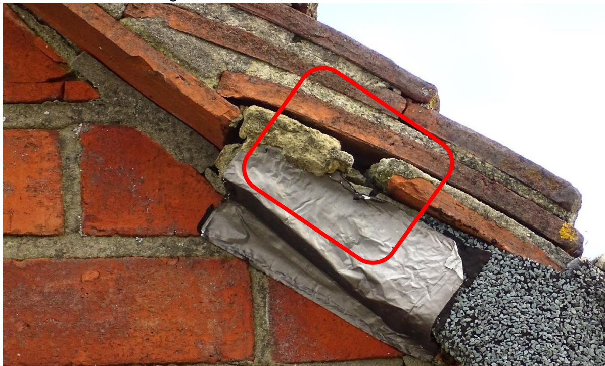
Image 5 Gaps within the roof coverings of proportion to offer daytime roosting value to crevice dwelling bats
