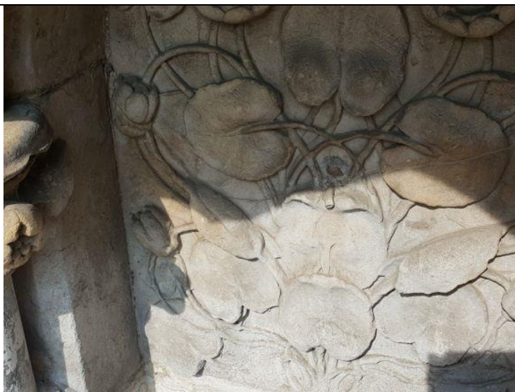
Fig 9. Top panel showing an example of failed pointing. It needs to be cut out by hand and repointed in soft lime mortar. (RBC. 2020)
