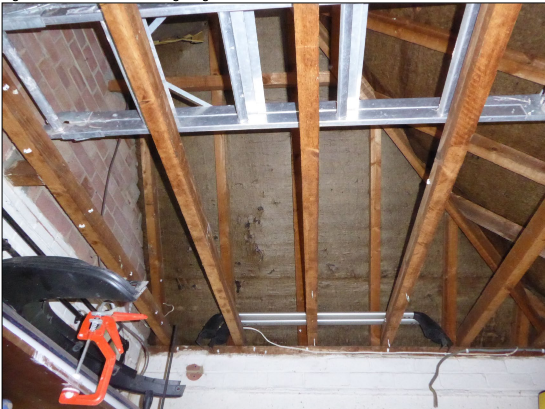
Figure 11. Internal view of garage roof. 3 Eric Avenue, Emmer Green. 05.06.20
