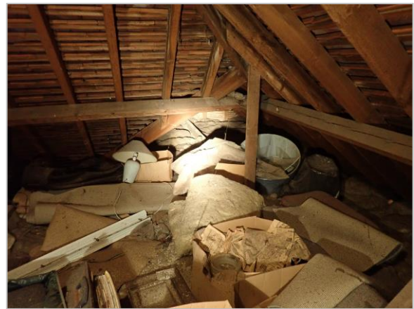
Photo 4 General conditions in loft
