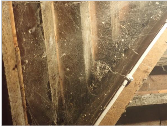
Photo 13 Heavy cobwebs across hip ridge beam
