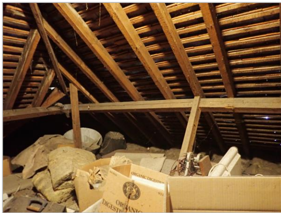
Photo 3 General conditions in loft
