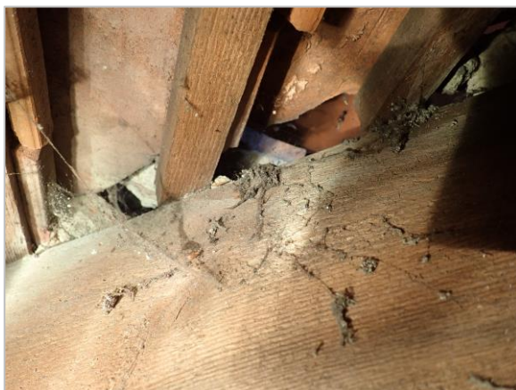
Photo 11 Ridge beam below ridge tile cavities
