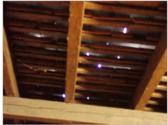
Photo 8 Small points of light visible between tiles
