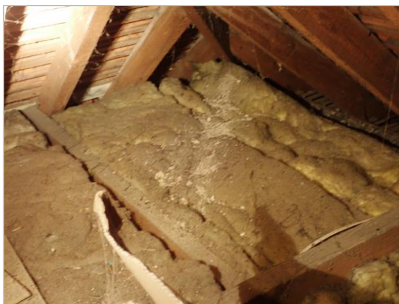
Photo 9 Line of crumbled mortar from hip ridge above
