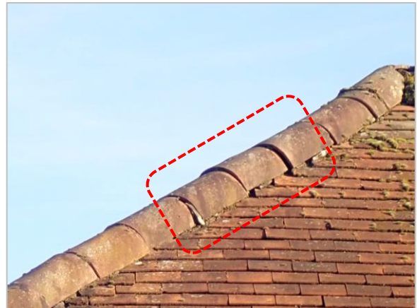
Photo 16 Missing mortar to hip ridge tile (see also Photos 9 and 10)
