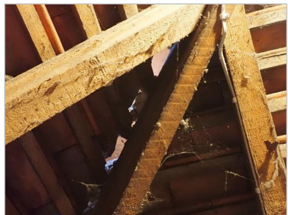
Photo 10 Exposed underside of hip ridge tile
