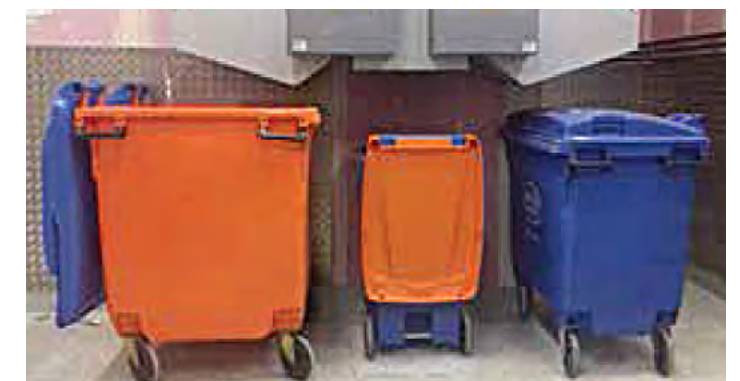
Tri-separator refuse chute
