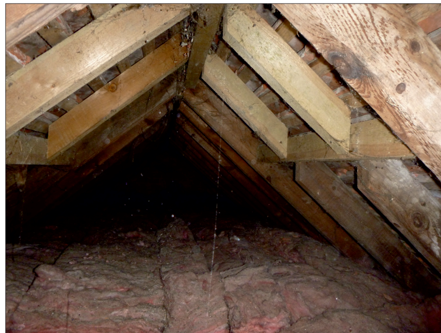
Photograph 4: Showing one of the restricted attic spaces, which was unlined and heavily dusty and cobwebbed throughout.
