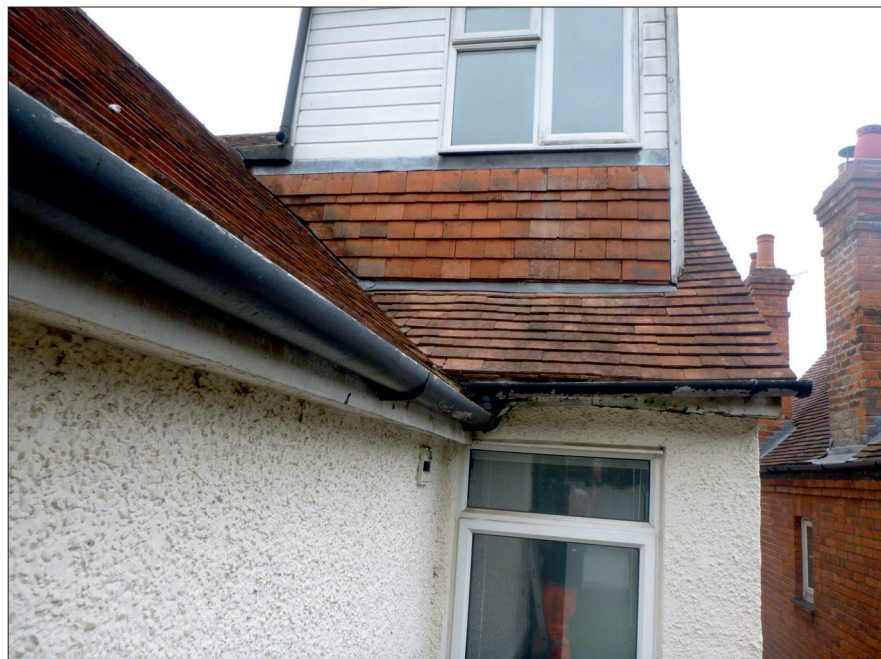
Photograph 3: Showing the restricted area of tile hanging on the bottom of the rear dormer.
