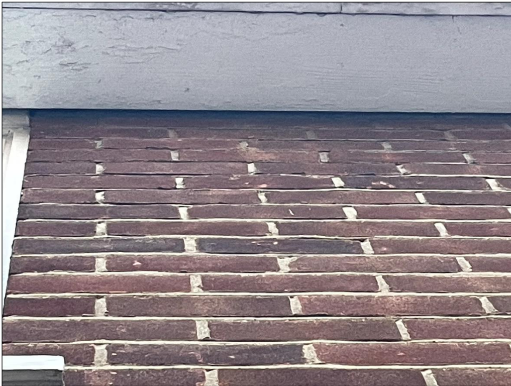
Plate 4. Gaps at soffit boxes
