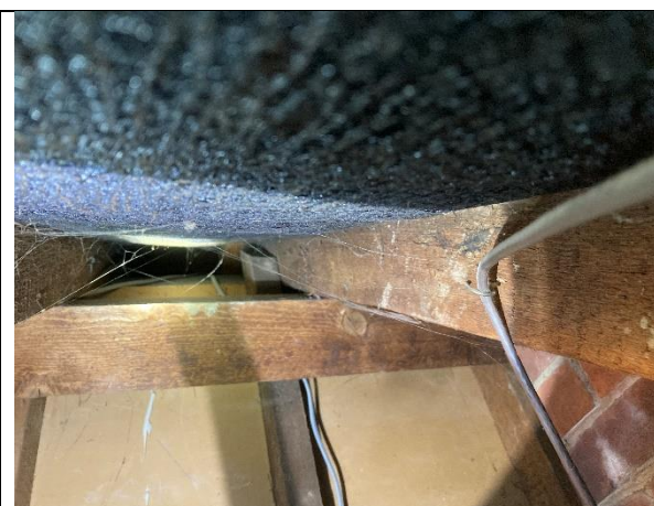
Photo 12 Example of cobwebbed void between vaulted roof and felt
