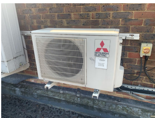
Fig 9: Wall mounted condenser to be retained, serving the ground floor offices
