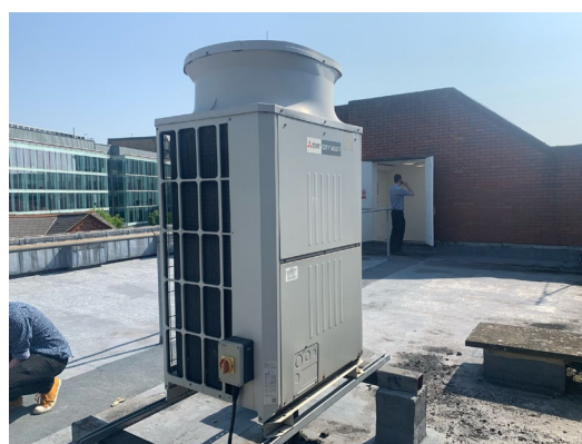
Fig 10: Floor mounted condenser to be retained, serving the ground floor offices
