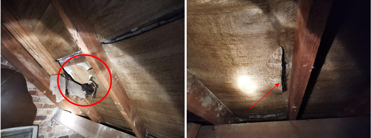
Figure 13. Example of tears/cuts in the roofing felt
