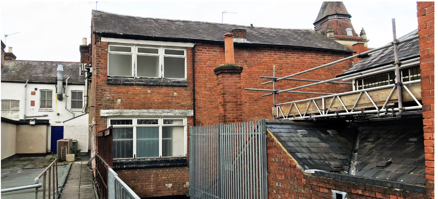
Rear of the existing building, which has been neglected and has degraded over time
