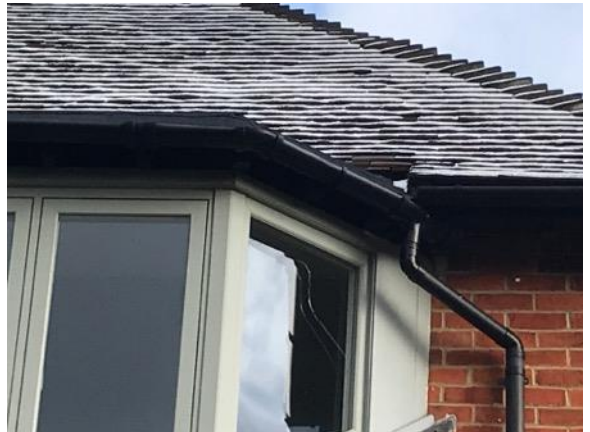
Photograph 6: Gap under tiles behind bay window
