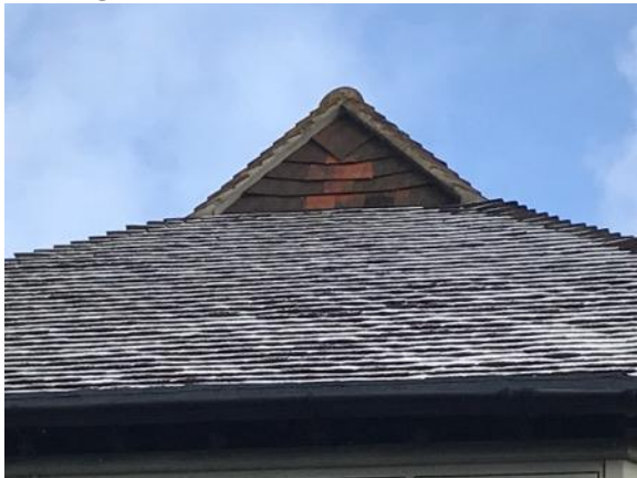
Photograph 5: Raised hanging tiles on the building
