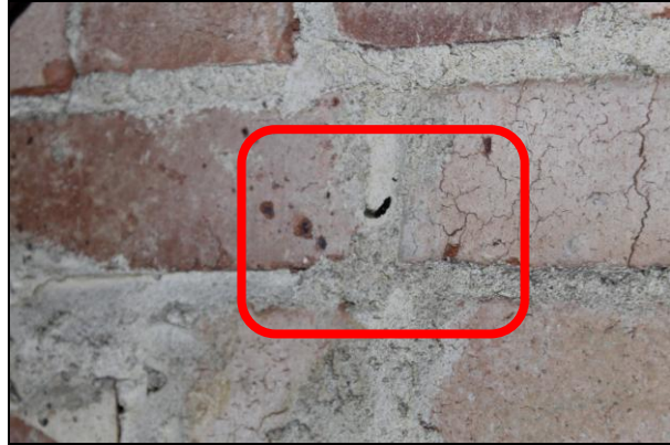
Plate 6: View of bat dropping adhering the internal dividing wall at the chimney breast
