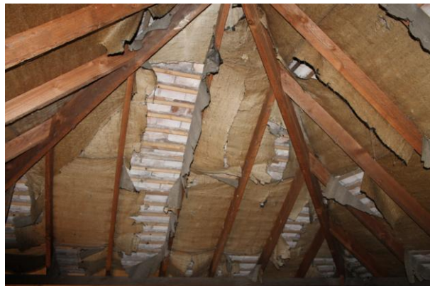
Plate 4: View of the underside of the roof interior showing the degraded nature of the felt lining
