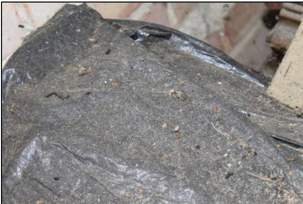
Plate 7: View of droppings collected near the internal dividing wall within the loft
