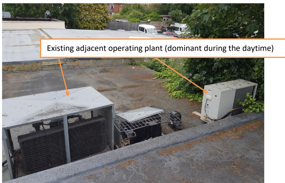
Figure D2 – Photo highlighting adjacent commercial rooftop plant (clearly audible in operation at position 1).
