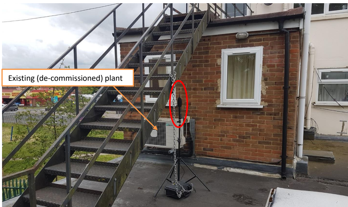
Figure D1 – Photo highlighting Measurement Position 1, showing de-commissioned condenser plant servicing the previous ground floor commercial use in immediate vicinity of the residential window.
