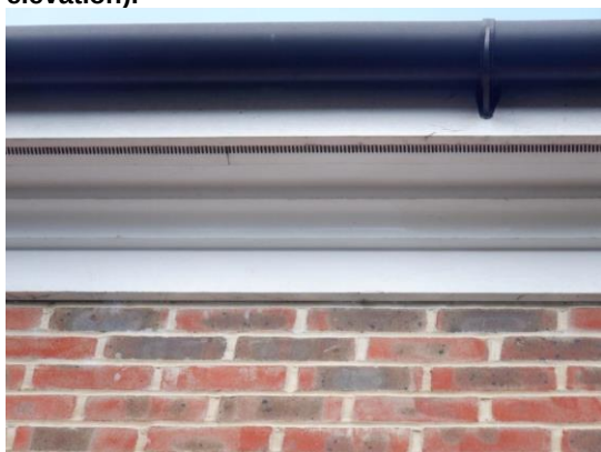
9. Soffit box tight against brickwork (rear elevation).
