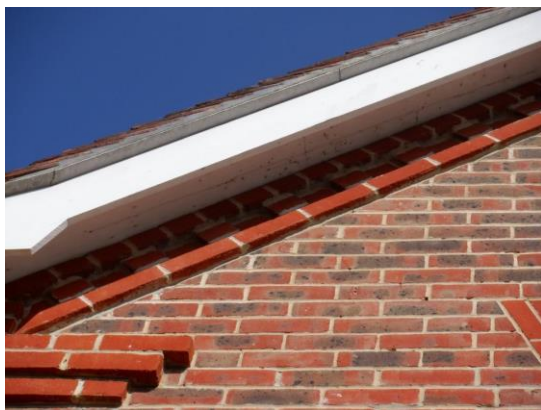
7. Intact verge mortar on front gable (front elevation).
