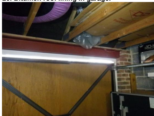
22. Gap along top of garage door.
