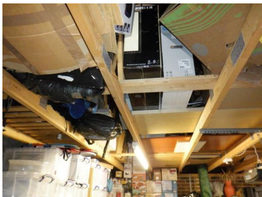
19. Stored items on joists in garage.
