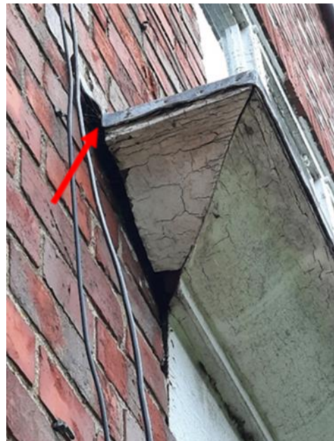
Plate 4.14: Gap behind wooden lintel and lifted lead flashing
