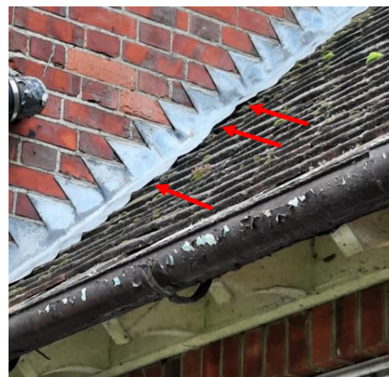
Plate 4.8: Lifted lead flashing between kitchen extension roof and main building
