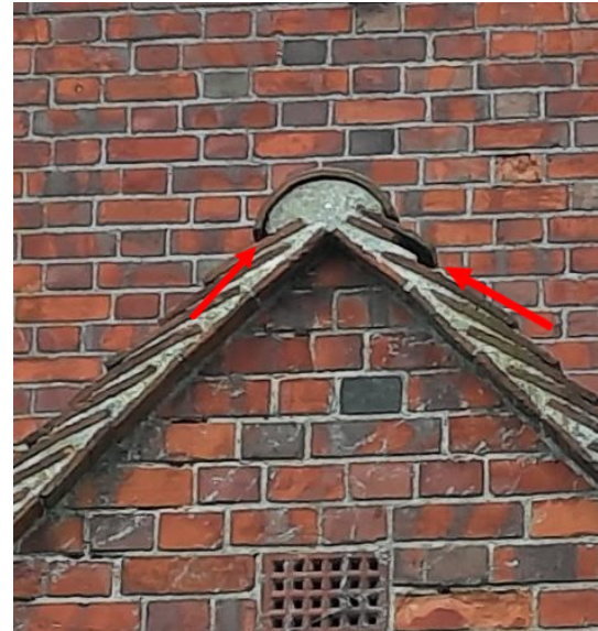
Plate 4.6: Lifted roof and ridge tiles on kitchen extension gable end
