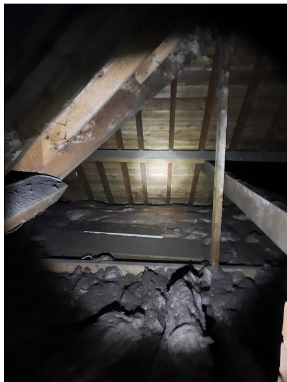
Plate 4.16: Main loft void – heavy cobwebbing
