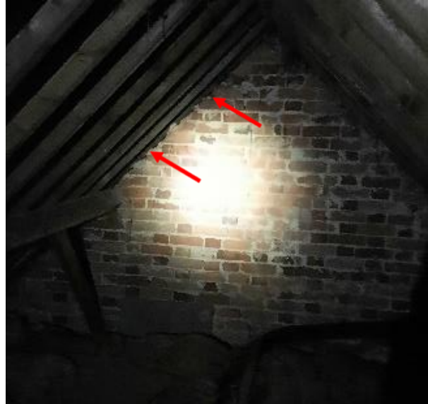
Plate 4.18: Gaps around most northerly rear gable end
