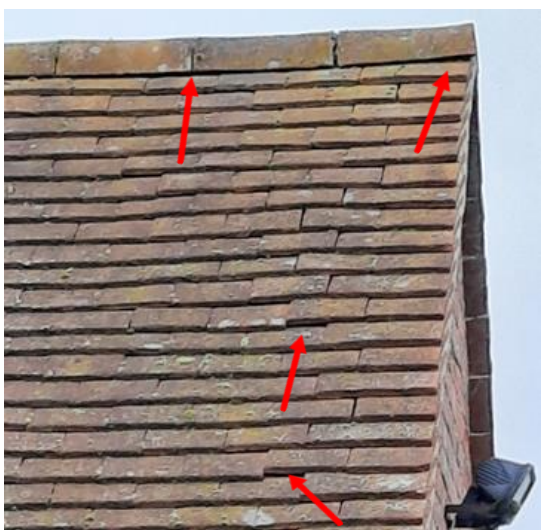
Plate 4.7: Lifted roof and ridge tiles on kitchen extension roof
