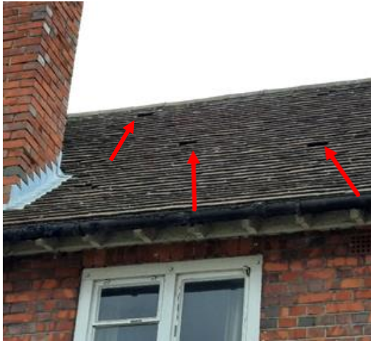
Plate 4.3: Numerous missing and lifted roof tiles (north-west elevation)
