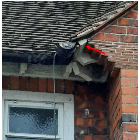
4.10: Gaps between wooden board and brickwork
