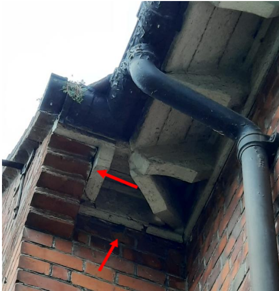
Plate 4.9: Gaps between wooden board and brickwork
