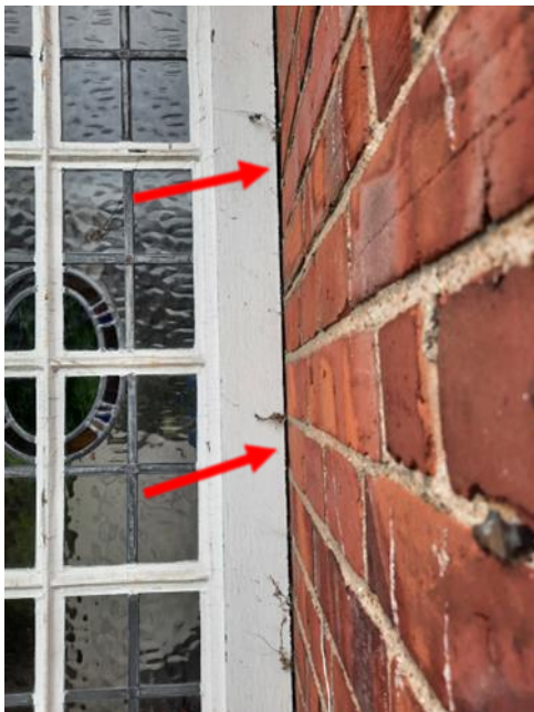
Plate 4.13: Gap between window frame and brickwork
