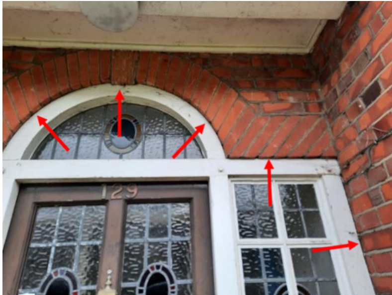
Plate 4.12: Gaps between wooden door/window frames and brickwork
