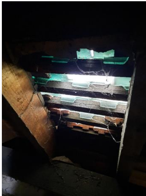
4.19: Broken roof tiles and missing sarking
