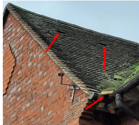
Plate 4.4: Missing and lifted roof tiles (south-east elevation)
