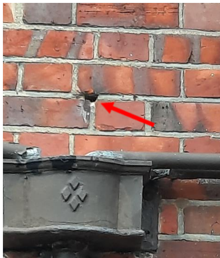
4.11: Missing mortar in brickwork (north-west elevation)
