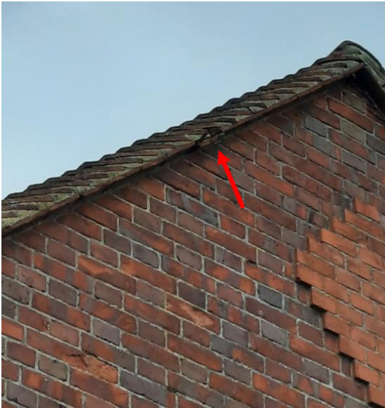
Plate 4.5: Broken tiles on gable end (north-east elevations)
