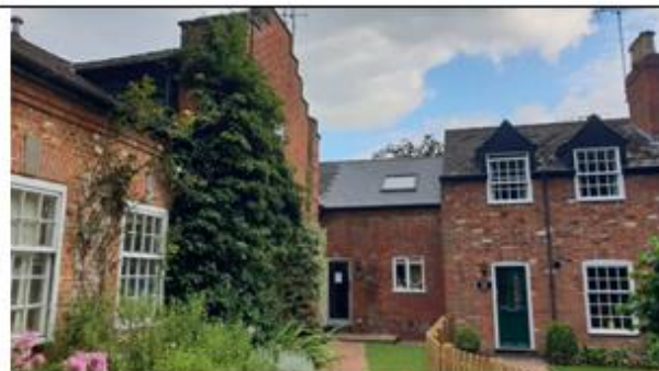
Fig 1: Entry to Cottage (8 The Brookmill). There is currently a mix of old and new slate tiles on roof.
